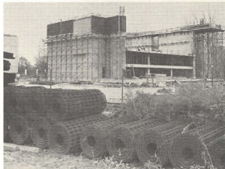
ROLLS OF REINFORCING WIRE await installation in the Library-Administration building. Rectangular structure on extreme left will be part of the completed building as shown in the rendering.
